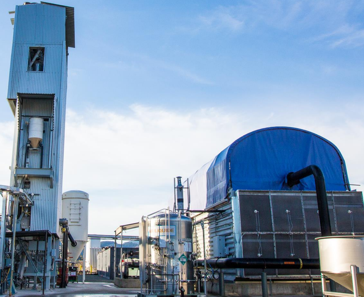
CE'S DIRECT AIR CAPTURE PILOT PLANT, SHOWING THE CALCINER & AIR CONTACTOR
